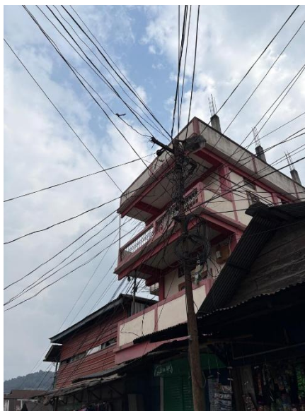
Fig. 19: Congested Electricity Pole and Overhead Wiring
